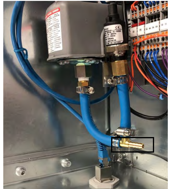
Image 4 – Air hose nozzle in power box
