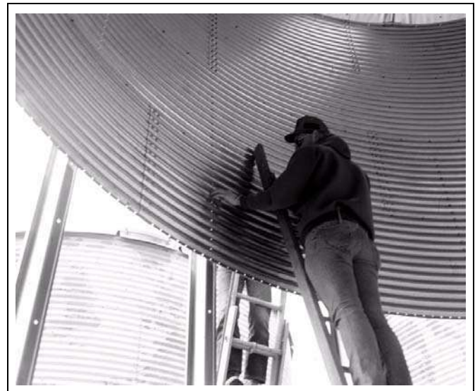
Figure 12H Installing legs to bin with bolt heads on the inside of bin and nuts on the outside.
