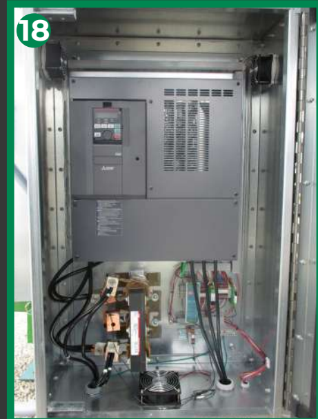
DC shield removed to show detail
