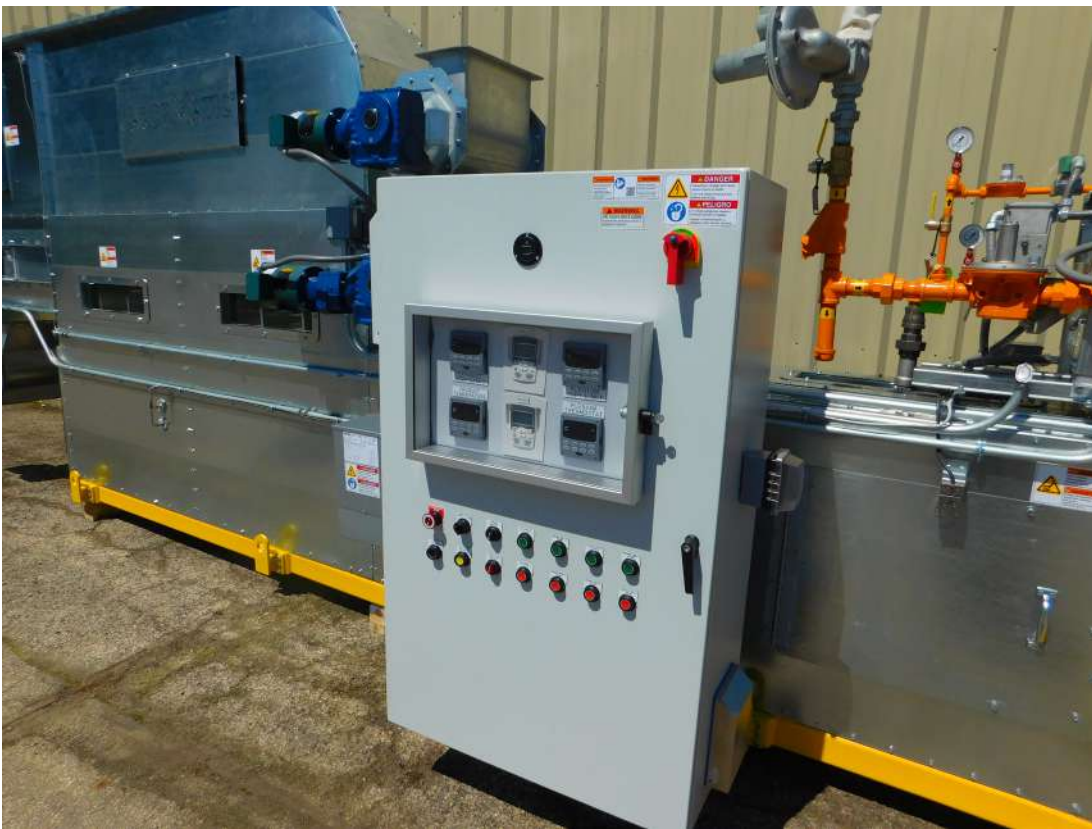
Control Panel Assembly
